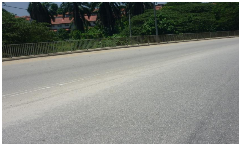
Rajah 26 : Faded Road Marking
